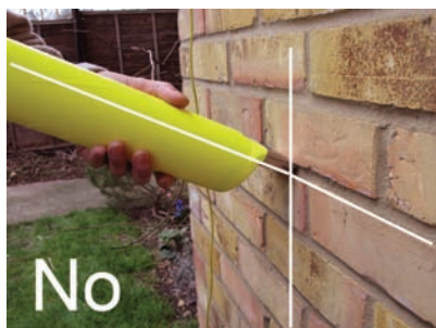
2. Nozzle is incorrectly seated
